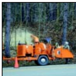
Roads Maintenance crew conduct right of way cleaning to ensure safe travel for County citizens.
