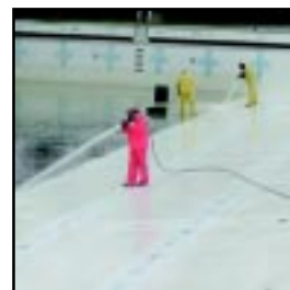
Parks Maintenance crew perform pressure cleaning, crack repair and painting as part of the annual preseason preparation at South Park Pool.
