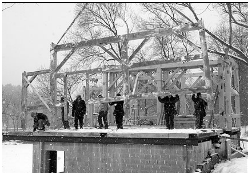
Amish workers from the Amish Timber Framers of Doylestown, Ohio erect framework on new barn.
