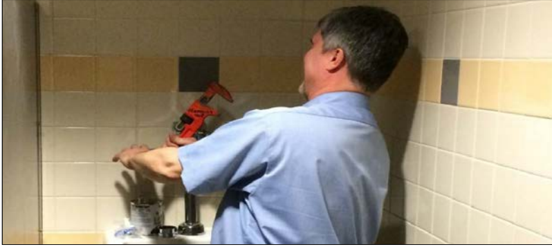
Fixing and upgrading bathroom plumbing at the County Office Building (Allegheny County Photography)
